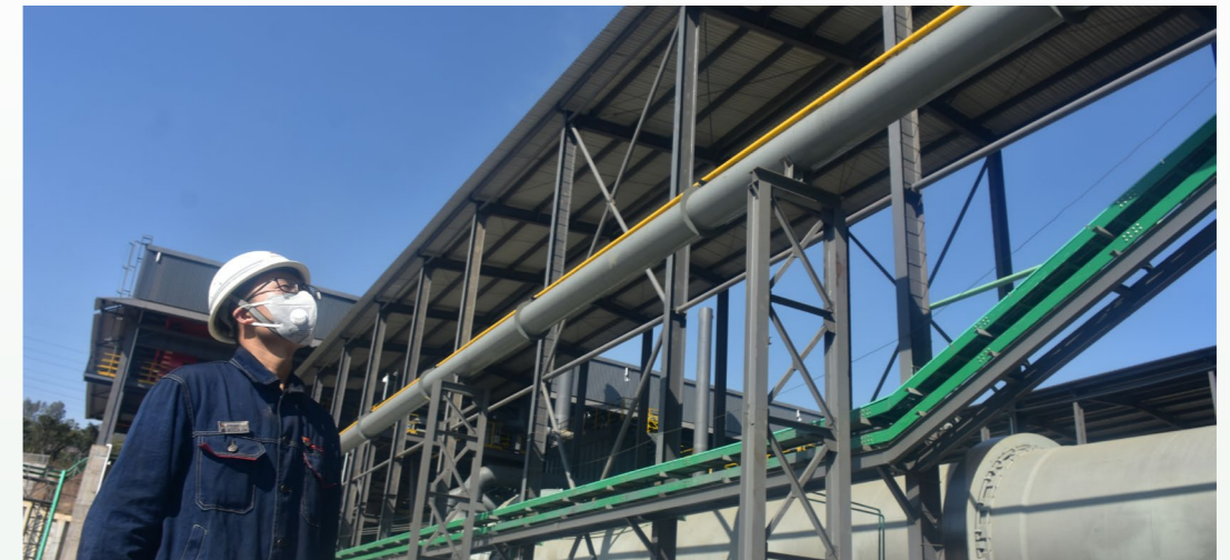
钛渣电炉煤气回收用于干燥湿钛精矿 Titanium slag electric furnace gas recovery for drying wet ore in drying kiln
