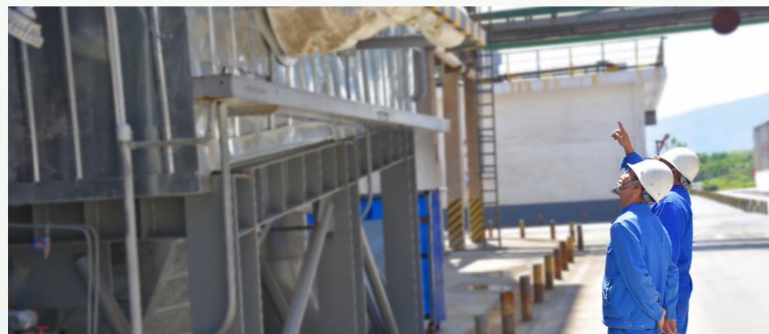
东方钛业员工查看闪干余热利用装置 The flash drying waste heat utilization facility at Dongfang Titanium Industry
