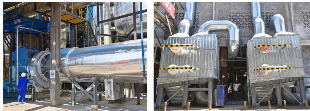
东方钛业员工查看钛液 MVR 蒸发浓缩系统 An employee of Dongfang Titanium Industry inspects the MVR titanium liquid evaporation and concentration system
